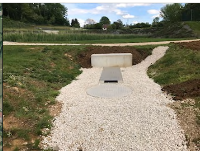
Station de traitement – Bannes Village
